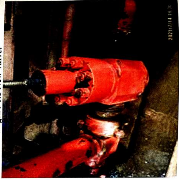
Figure 6.2 Valve to be replaced
