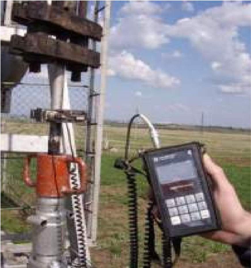
Figure 2 (b). Installed dynamometer
