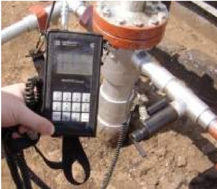
Figure 2 (a). Installed echometer
